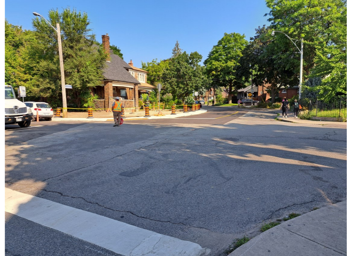
Photo: Road restored for vehicular/pedestrian traffic at Linnsmore Cres. and Strathmore Blvd.
