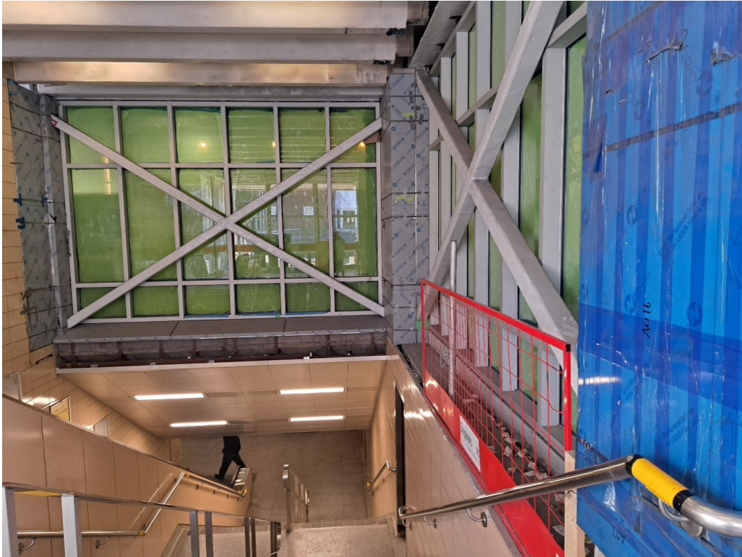
Photo: Ceiling panel and light fixtures installed at street level (inside the station view)
