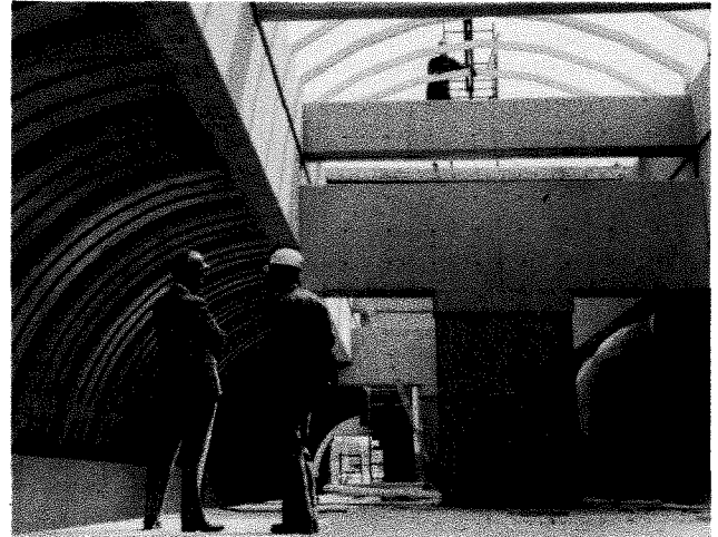
Glencairn Station — platform level. The open area above will contain a 180-foot long glass skylight.
