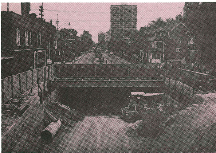
Work is continuing at a good pace on the 6.17-mile Spadina Subway. The open-cut section on Spadina, between MacPherson and Lowther is pictured above. View looks south to main intersection of Dupont and Spadina. Soon the wooden decking will be removed and the road repaved while construction continues beneath the street level.
