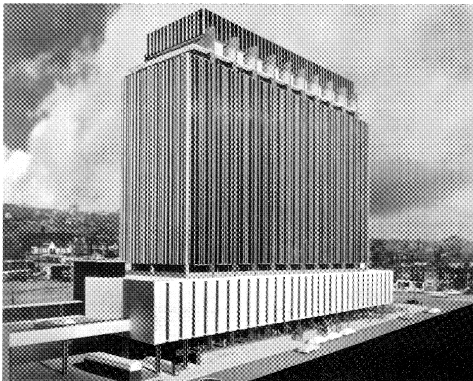
Latest addition to the many fine commercial and office buildings erected in the Eglinton-Yonge area since the Yonge subway was built is the 17-storey office building shown above which is now under construction over Eglinton subway station. It is scheduled for completion in March 1963.
