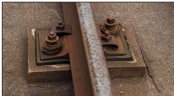
Figure 19 - Typical Track Fastener Assembly at Accident Site
