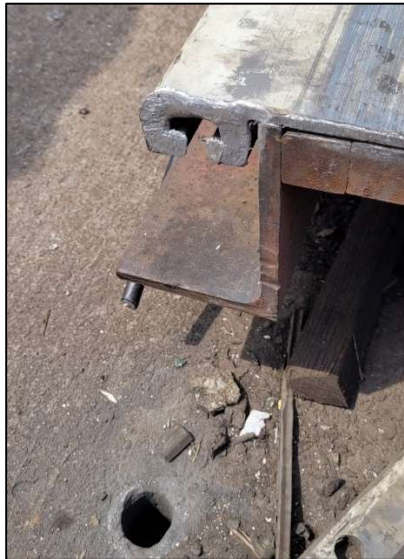
Figure 27 - Damaged Aluminum Top Cap of Reaction Rail Section A
