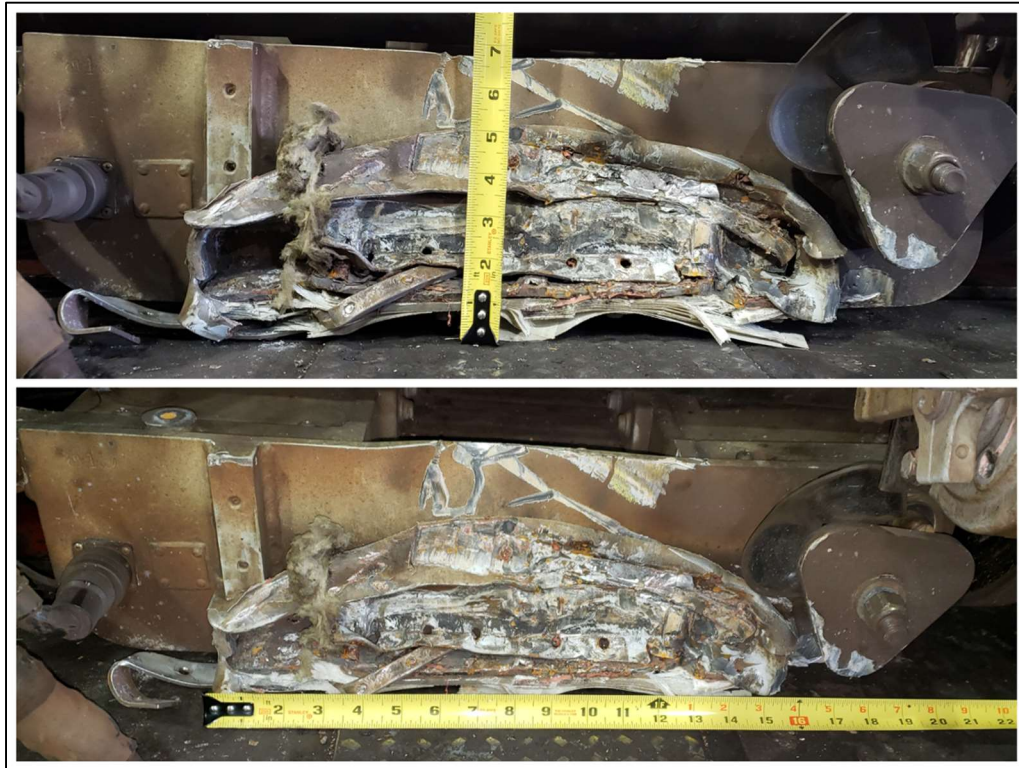
Figure 86 - LIM Damage on Truck S/N 020
