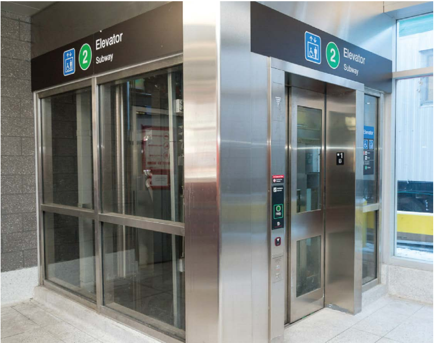
Image of a new elevator at Lansdowne Station
