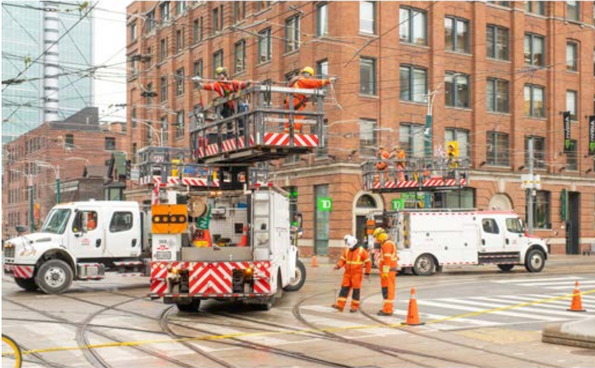
TTC overhead crews conducting emergency repairs at King St and Spadina Ave in December 2024.
