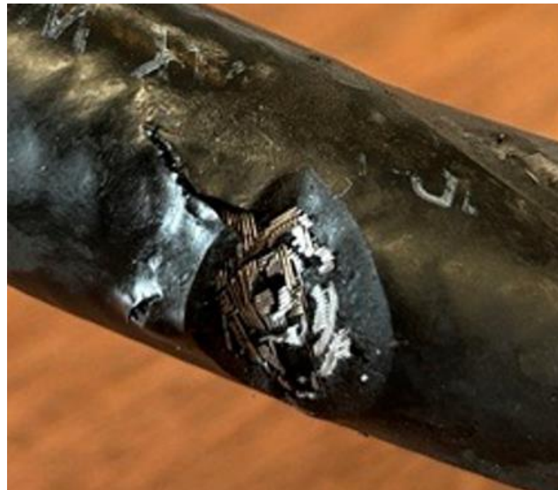
Above: Abraded hose on RT-56.
