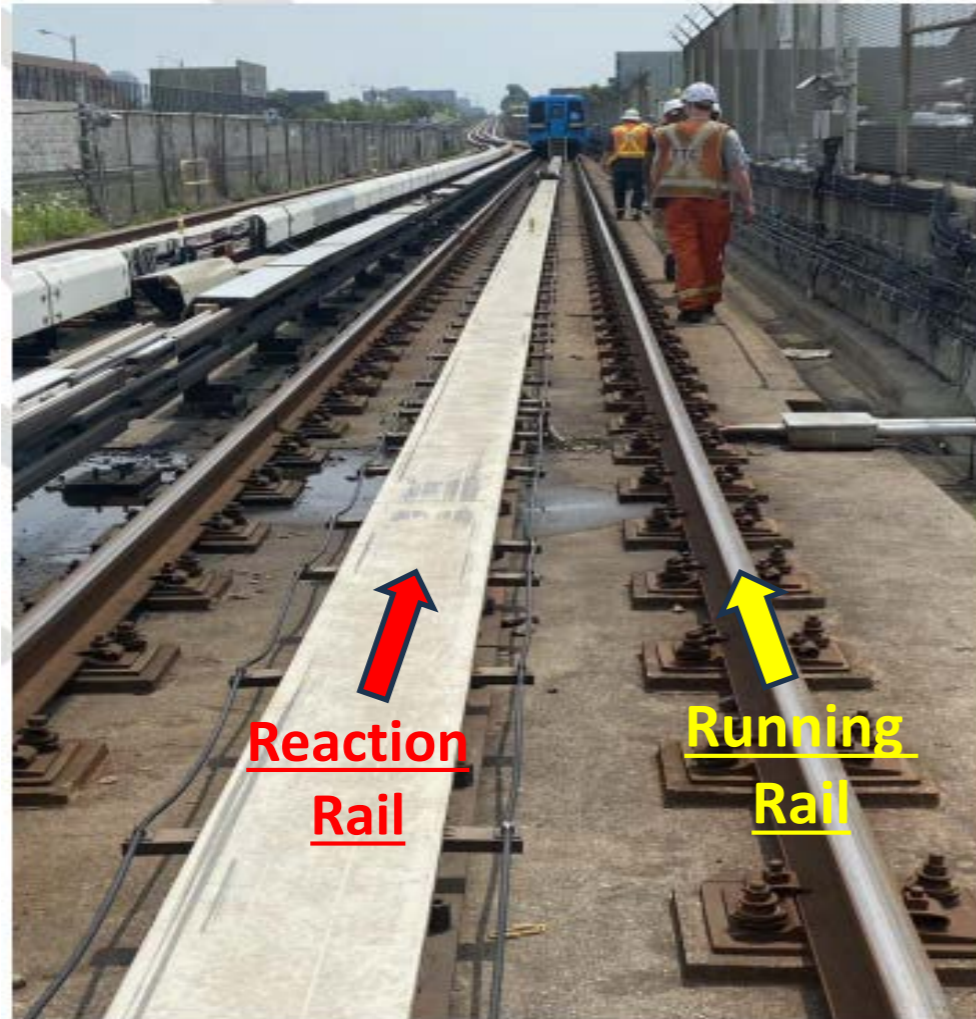
SRT Rail System
