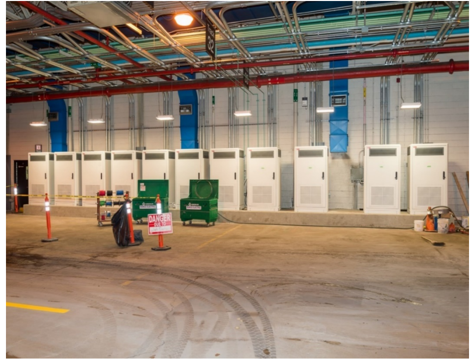
Photo of eBus charging stations (power and controls) at Mount Dennis Garage
