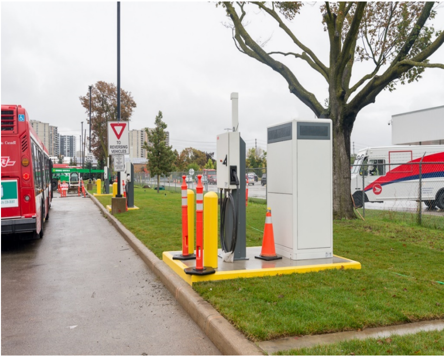
Photo of eBus charging stations (power and controls) at Mount Dennis Garage
