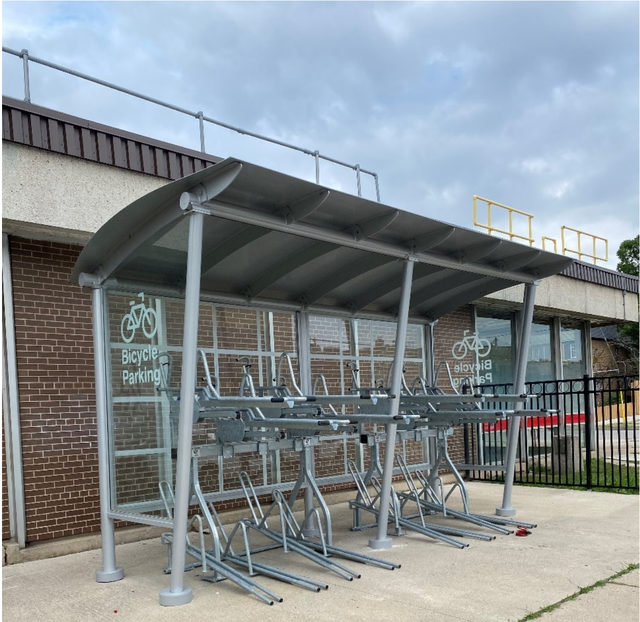
Figure 14: Bike shelter installed at Royal York Subway Station
