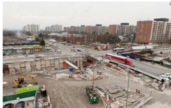
Finch West Station. Photo of Keele Street closure northbound at Finch Avenue West. Station box openings on both the south and north sides of Finch Avenue West
