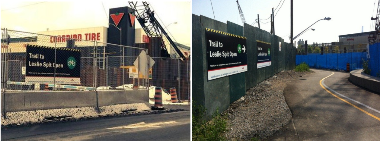
Cyclist signage on the south side of Lake Shore Boulevard at Leslie Street, the Martin Goodman trail remains open throughout construction
