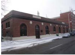
Exterior of the Danforth building indicating good visibility and a positive historic character.
