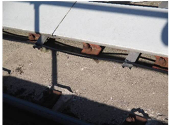
Figure 3: Broken anchor bolt
