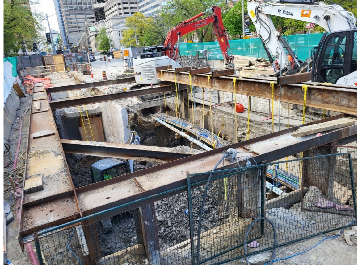
Excavating the elevator shaft on west side of Queen’s Park, looking north.
